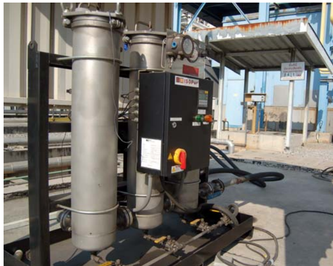
Figure 2. ISOPur HR Filtration Unit in Service
